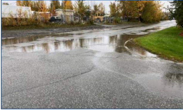
Flat grades & heaved curbs result in ponding at the Quinhagak Street & E. 63 rd Avenue intersection
