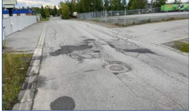
Significant pavement degradation with recent repairs along Quinhagak Street
