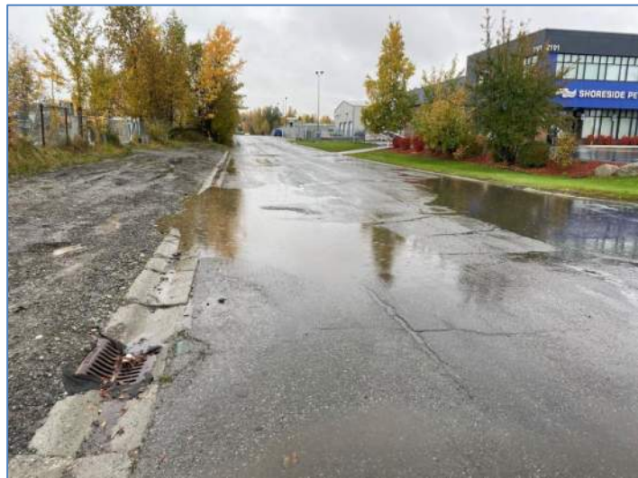
Widespread ponding & ineffective catch basin at the Quinhagak Street and E. 64 th Avenue intersection
