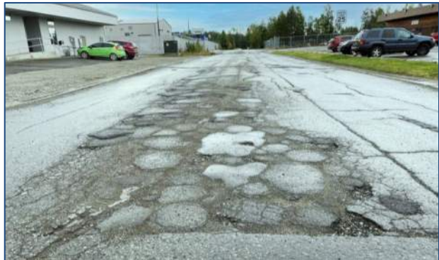
Poor roadway conditions along Quinhagak Street require regular attention from MOA Street Maintenance
