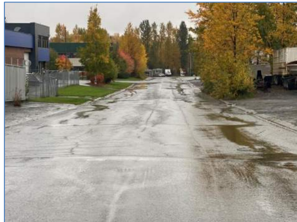
Heaving curb & gutter and ponding along Quinhagak Street (looking south)
